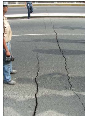
Figure 14. Cracking of the deck due to the January 5, 2006 event in the same structural section of the arch rupture. (January 5, 2006).
