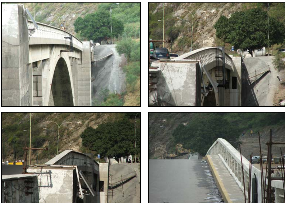
Figures 11a, 11b and 11c. Comparative views of deck deformation at different dates (August, 2005, December 2005, and January 5, 2005). Figure 11d: Closed view of deck vertical deformation which had reached 130 cm at the crown and 167 cm at the ruptured section; picture taken from the Caracas pilaster in March 9, 2006.
